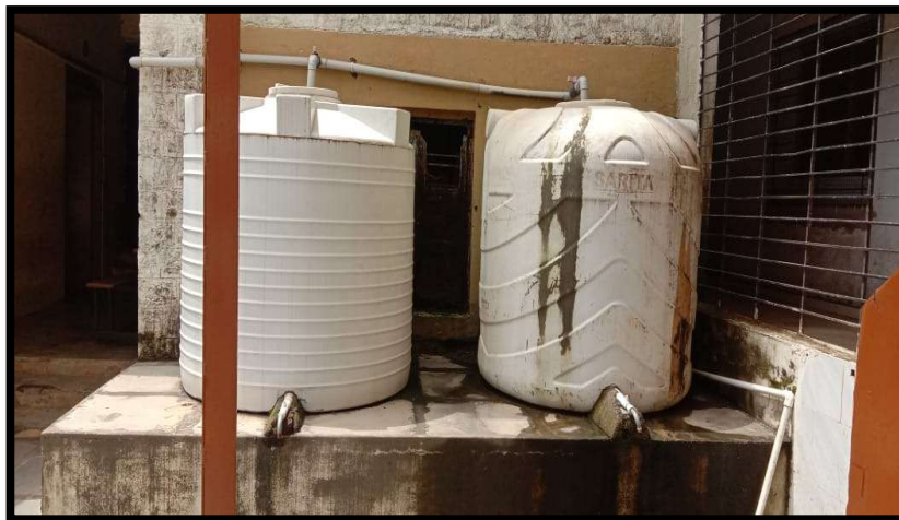
Rain water harvesting system provided with centralized storage tank in campus
